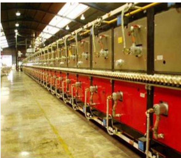
Furnace with 1500 rollers
